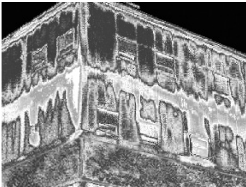
Testing shows energy loss despite insulated wall system
