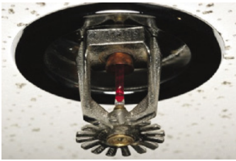
Fire sprinkler Tech.
