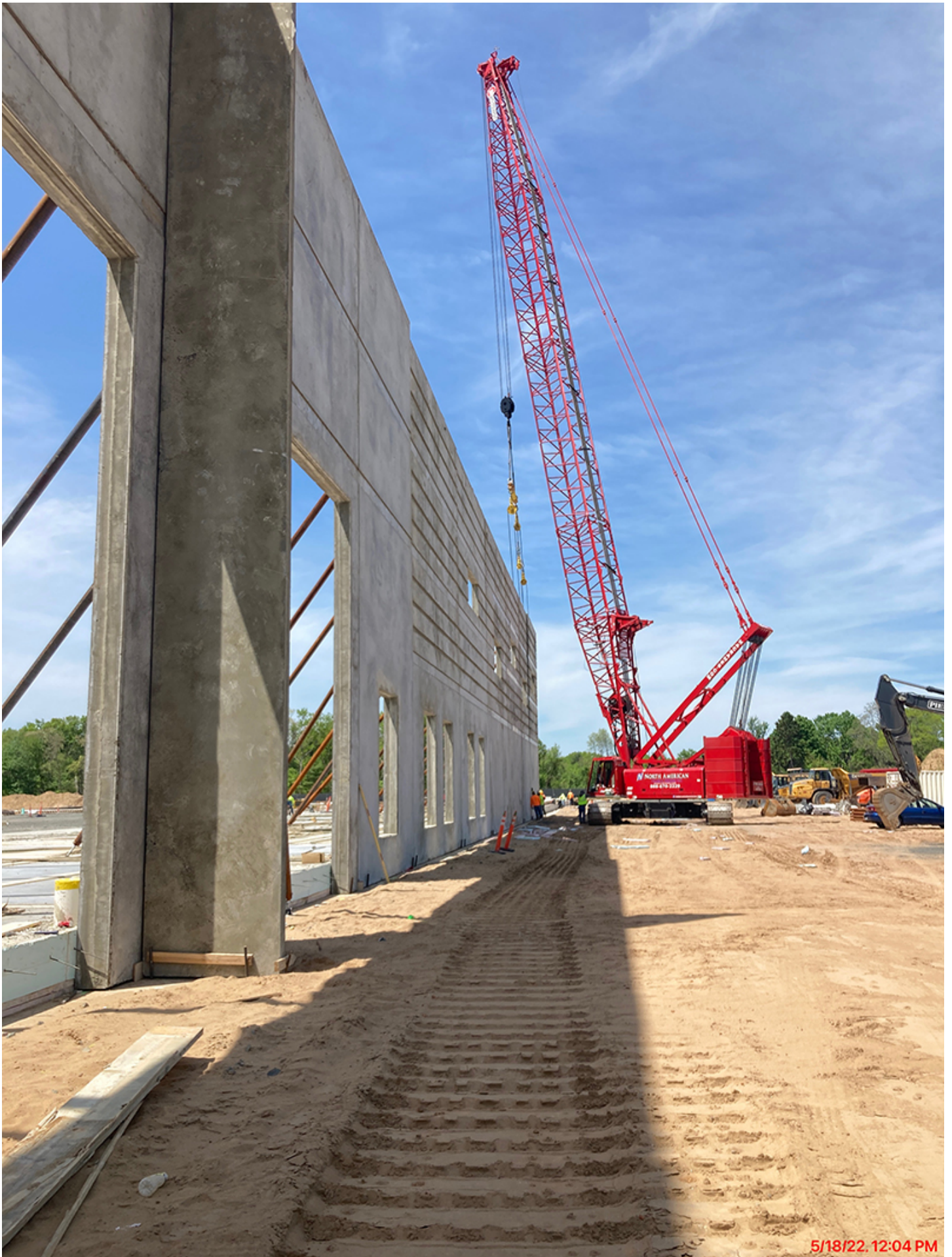
Windsor, CT According to Condyne Capital Partners and Polar Design Build tilt-up walls have been fabricated and erected for the Baker Hollow Logistics Center. All site work has been completed
