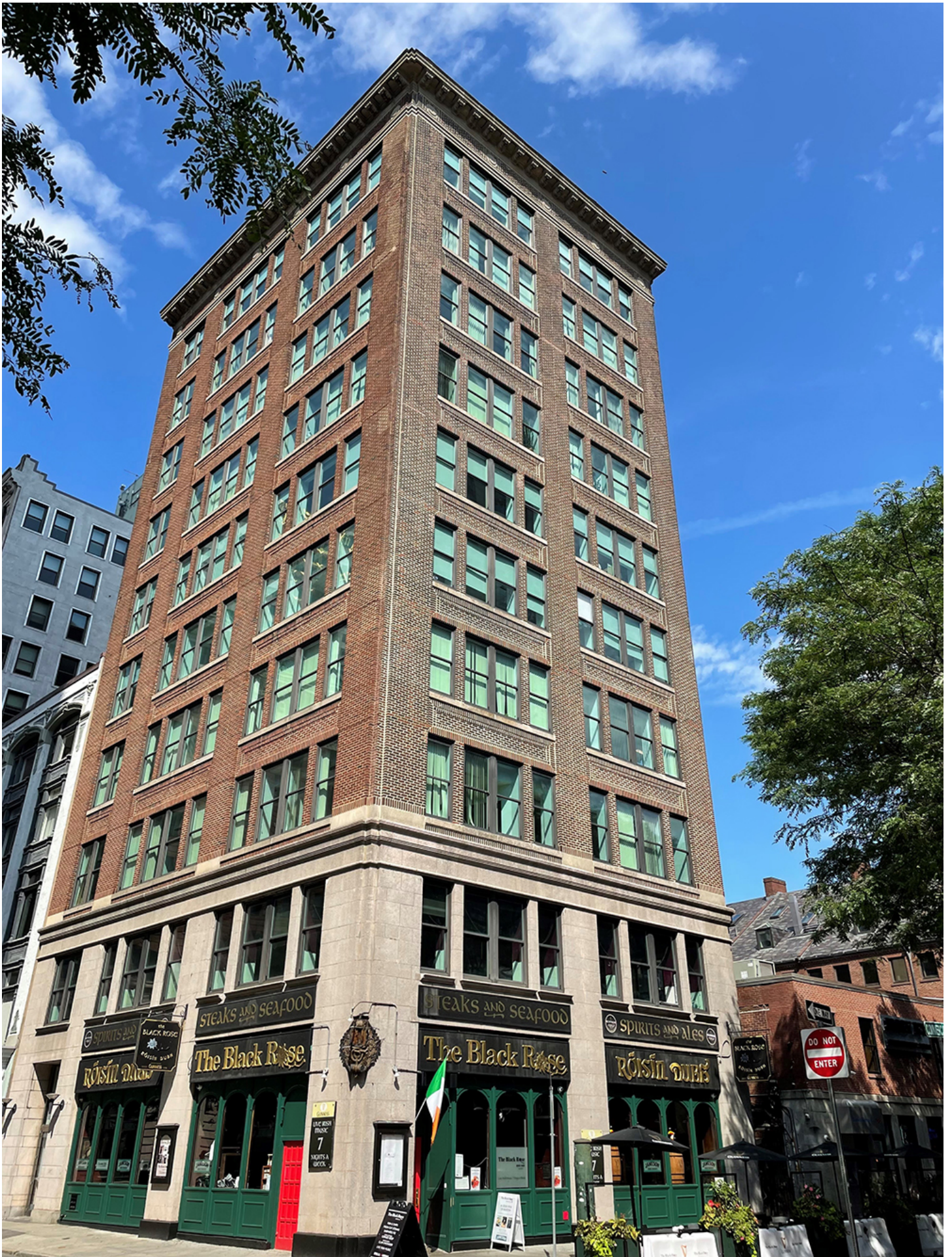
Boston, MA Abbot completed a comprehensive masonry repair project on a 10-story brick and concrete commercial/office building located at the corner of State and Commercial Sts. in the
