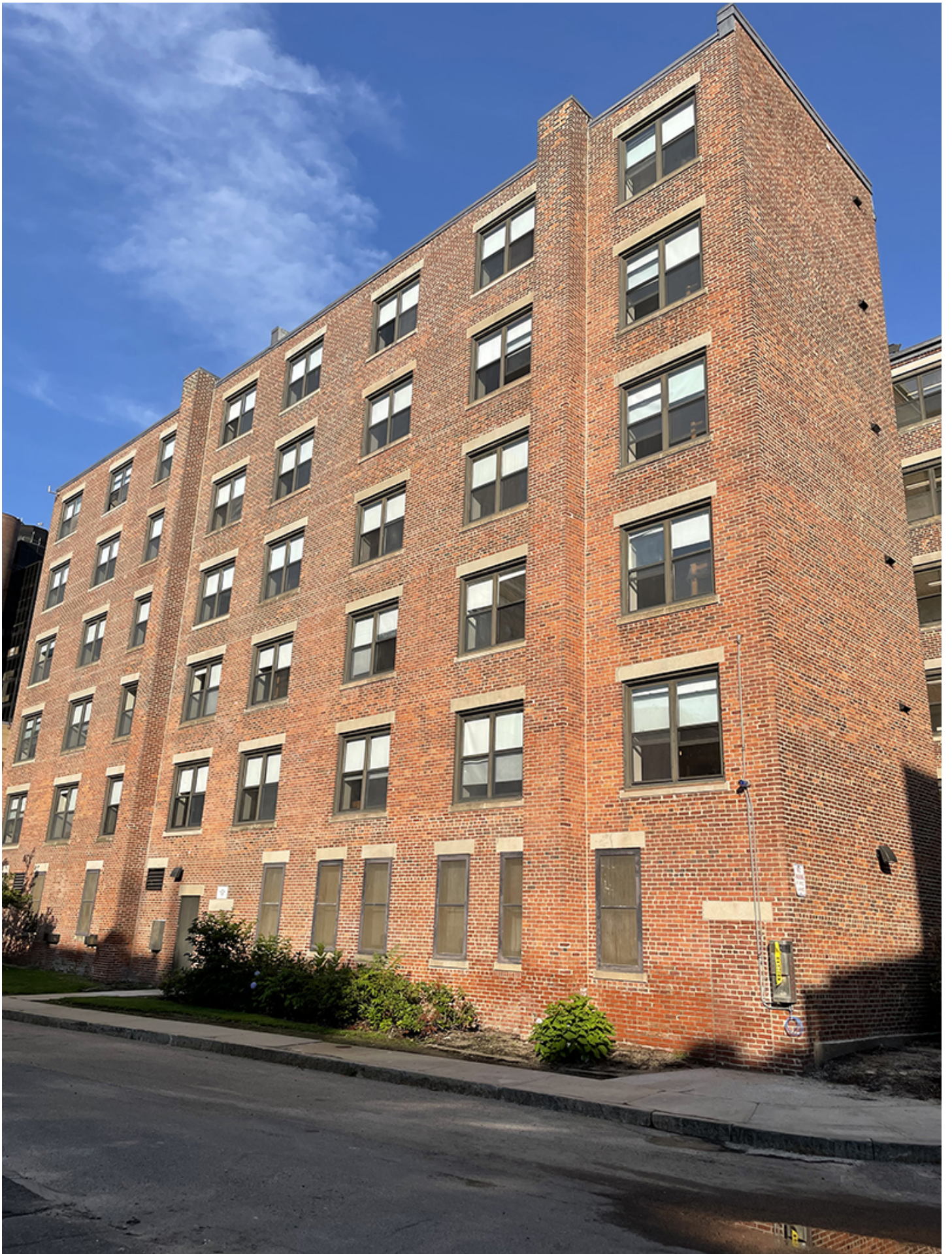
Boston, MA Abbot Building Restoration Company, Inc. has completed repairs on a four-story brick and precast concrete college dormitory building located on the campus of Wentworth Institute of
