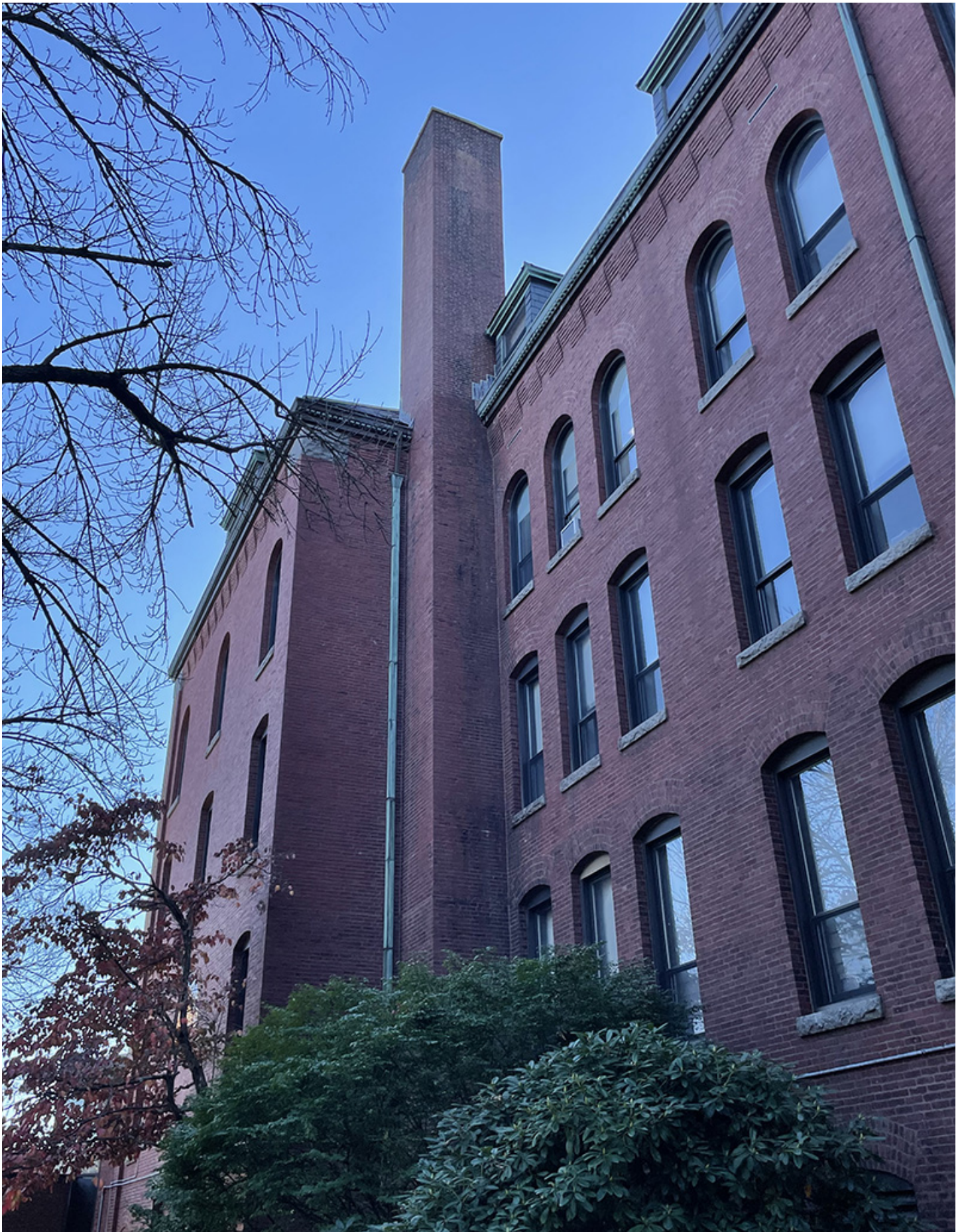
Newton, MA Abbot Building Restoration Company, Inc. has completed chimney repairs at the Leventhal-Sidman Jewish Community Center (JCC).
