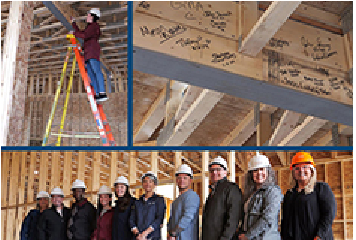
Shown are: Easterseals NH leadership and Gammon Academy School staff celebrate a beam signing event at the new Gammon Academy School building.
